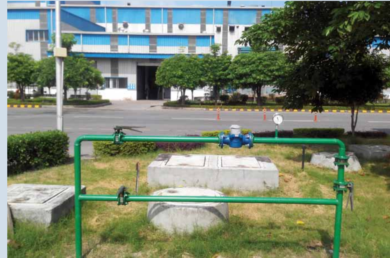
Flow meter at New Compressor House-Process
