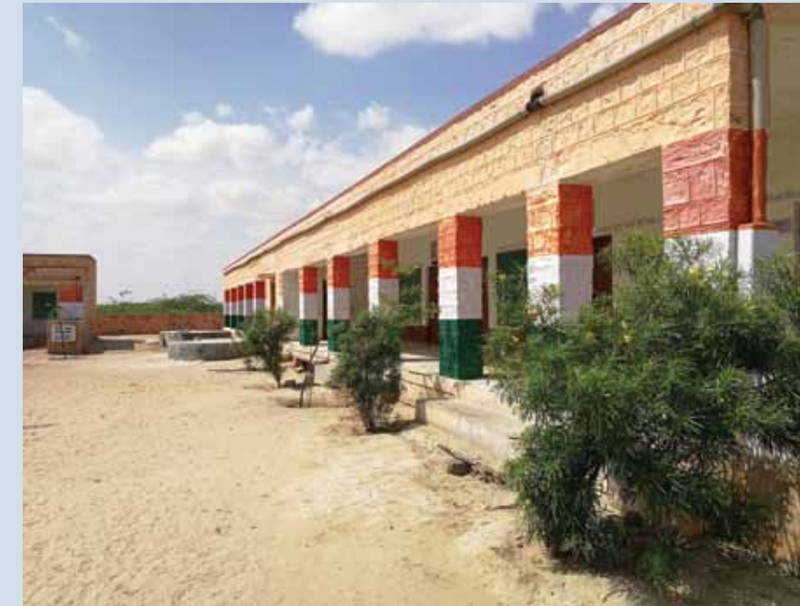
Roof water harvesting structures at Adarsh Dhunda School
