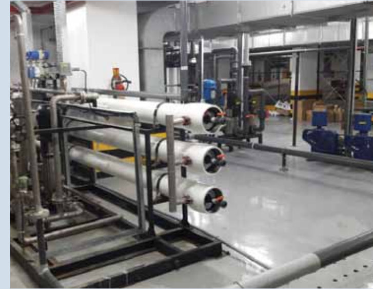
Water treatment plant, Reverse Osmosis
