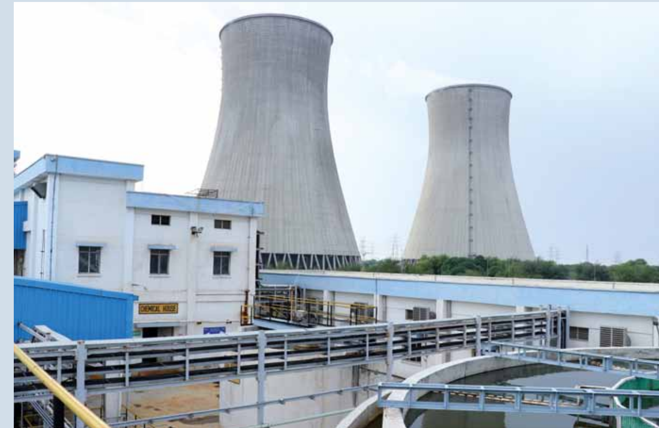
Natural Draft Cooling Tower
