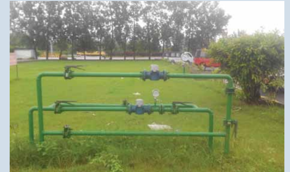
Flow meter Process and Drinking
