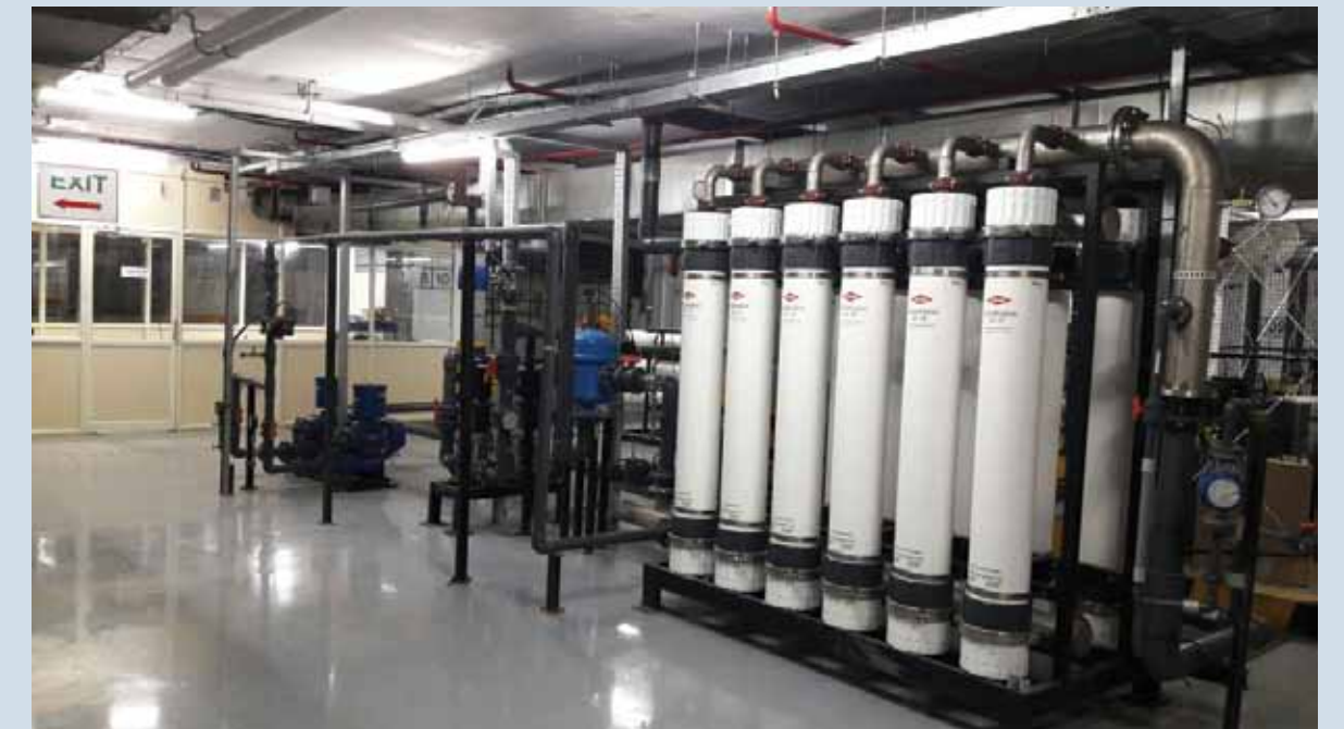
Water treatment plant, ultrafiltration
