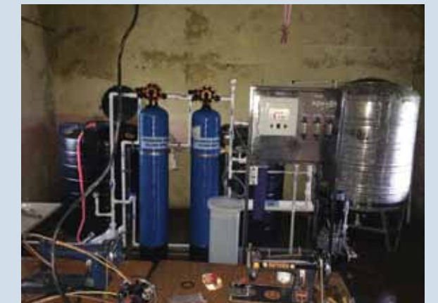
RO Plant, Bhawli, Igatpuri, Nashik
