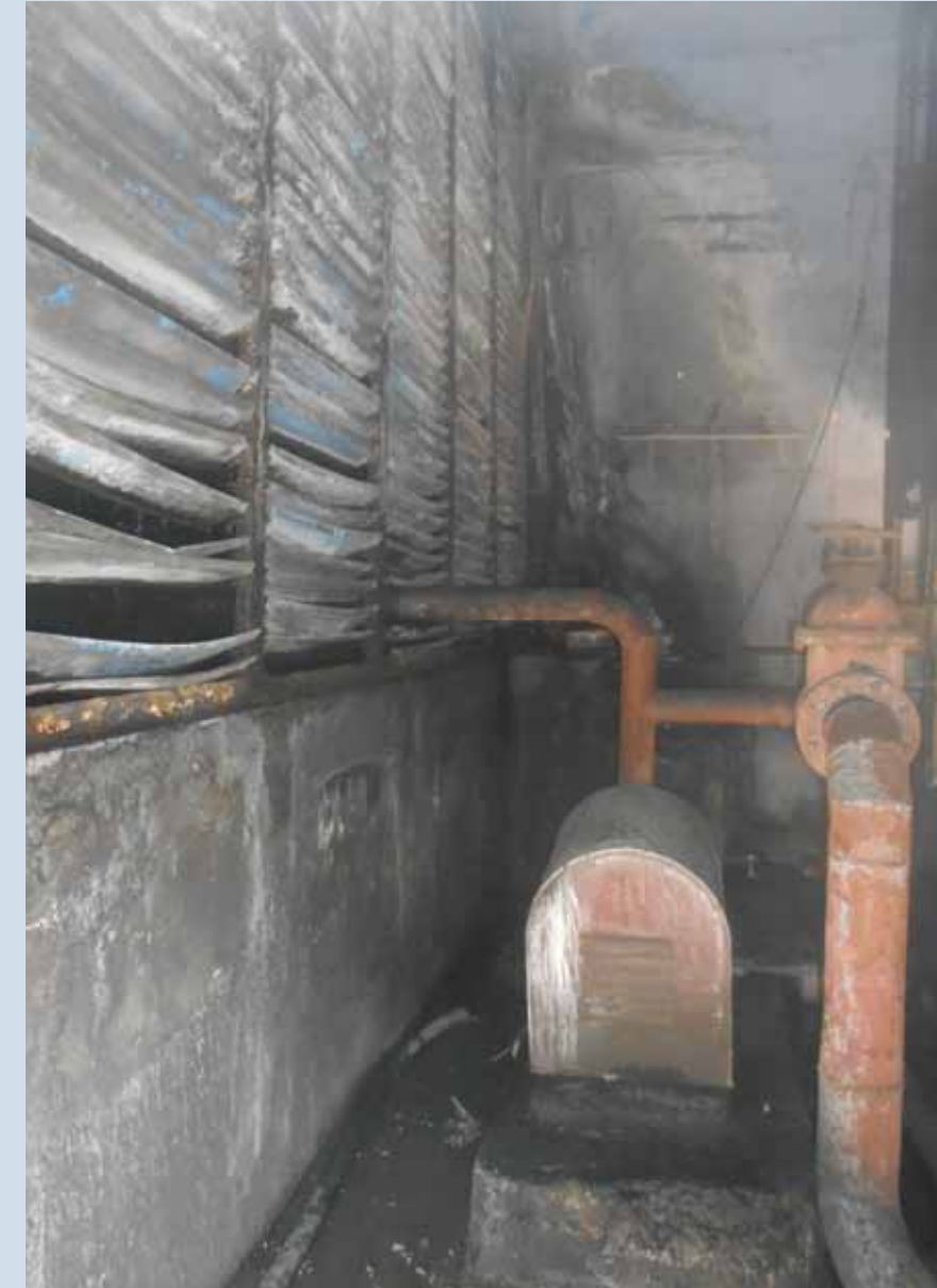
Water circulation tank
