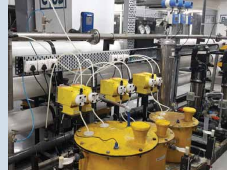
Water treatment plant, chemical dosing
