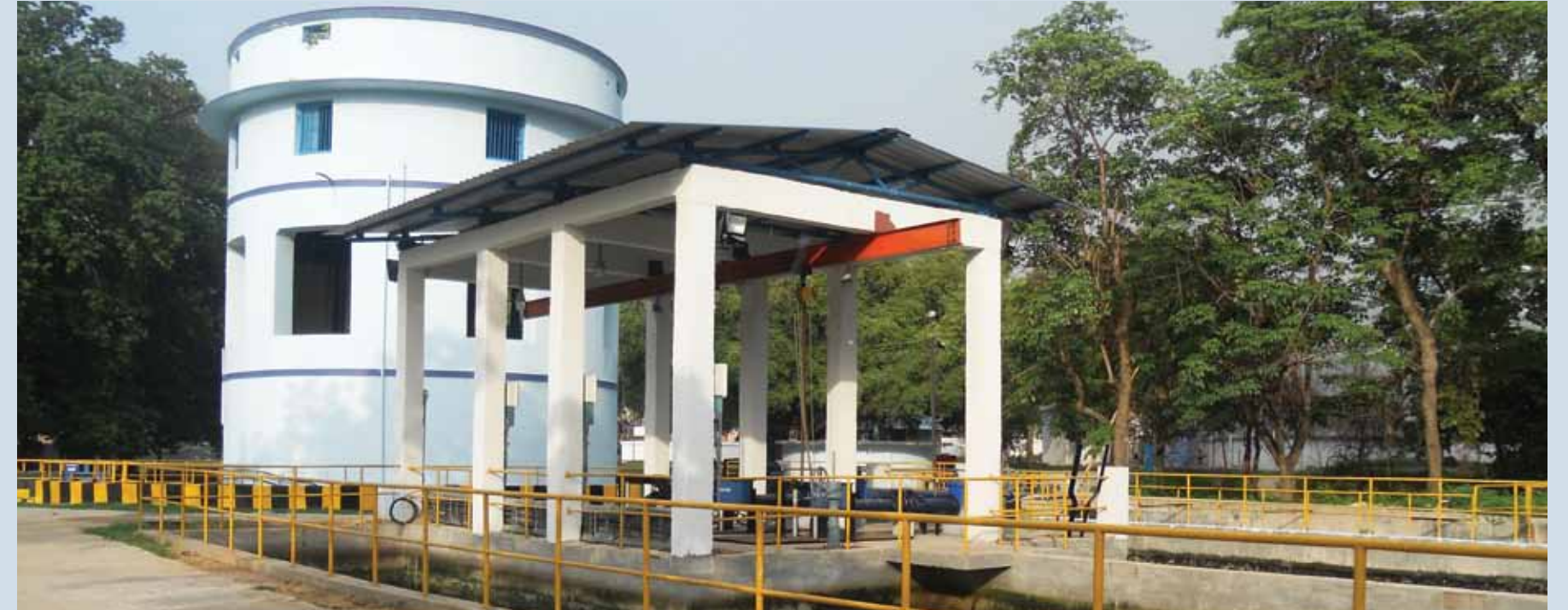
Reservoir treated water
