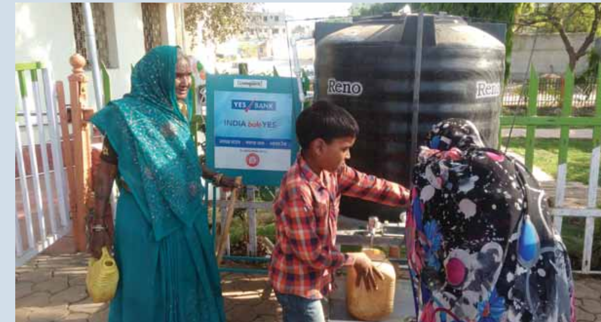
Drinking water system installed at D and E category railway stations
