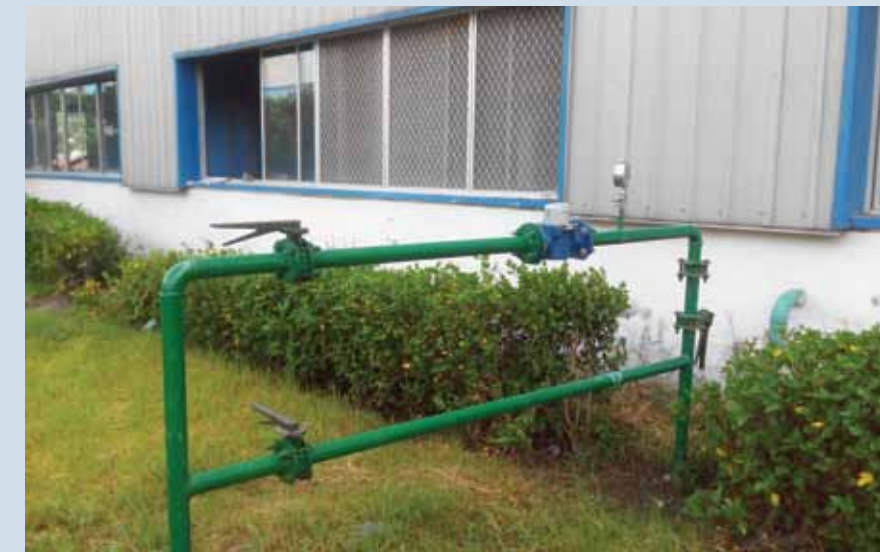
Flow meter Drinking
