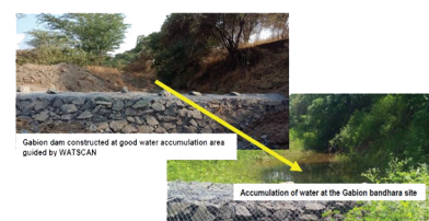
Gabion dam constructed at good water accumulation area guided by WATSCAN Accumulation of water at the Gabion bandhara site
