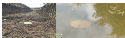
Implementation of trench & recharge shaft Recharge shaft submerged under water, for groundwater recharge.
