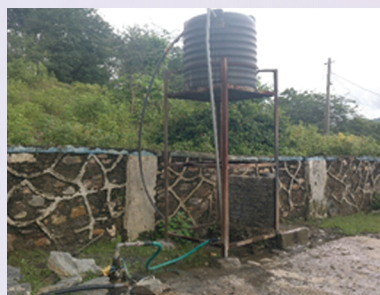
Drinking water supply at Borakheda village (Evaluation of water supply infrastructure)
